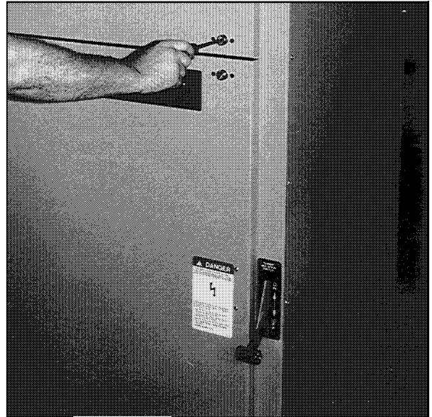
Fig. 38: Preparing For Initial Energization
