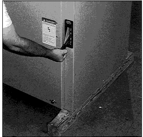
Fig. 39 Closing Isolation Switch
